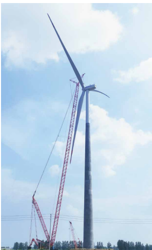
Steel Tower 90~120m
